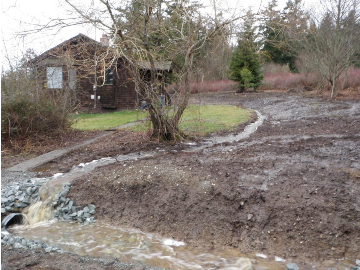
Figure 9. Ditch collecting flow just uphill of the caretaker house and conveying the water to the roadside ditch. Photo by Bruce Brown, 1/30/2013.
